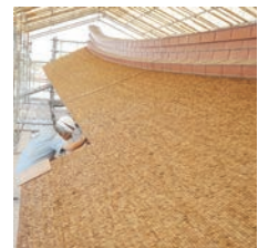
One of the privileges of working in restoration is to be close to parts of structures that are going to otherwise be inaccessible for decades to come and see details that will be invisible from the ground. A challenge for historic site preservation is inspection and timely maintenance.
